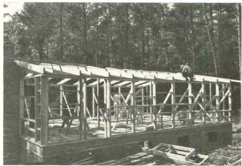
Construction is of framing panels preassembled in builders' yard of 3" x 6" posts rabbeted at sawmill. Trusses are two 2" x 8" spaced 4'-1/2". Ceiling is of 2" x 6" planks with roofing felt plus built-up roof. Overhangs are 2' or 3' on all sides. Roof pitch is 1 1/2 to 12.
