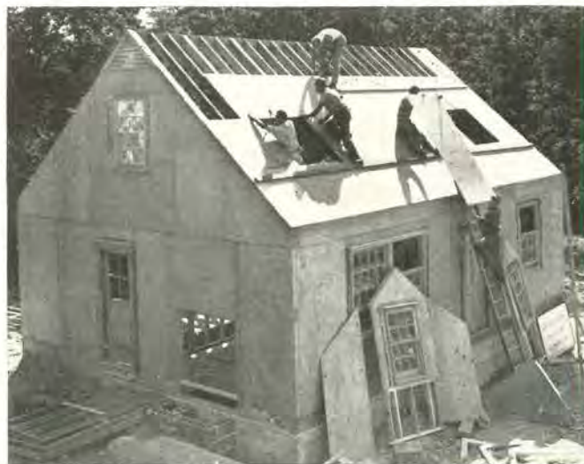
Roof goes on at 3 p. m. Six to eight men can erect shell of an average house in less than a day. Most firms supply roof trusses or pre-cut rafters.
