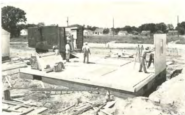
Bare slab at 8:00 a. m. Trailer parks at one corner, delivers wall panels which go up so rapidly that by late afternoon the house is completely enclosed, roofed and under lock and key.
