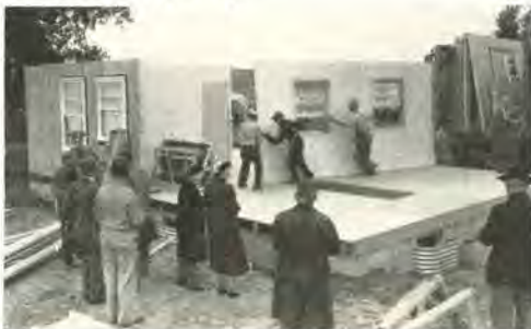
Houses that go up fastest are those with full-length panels and complete exteriors. Special equipment is often necessary to handle them.
