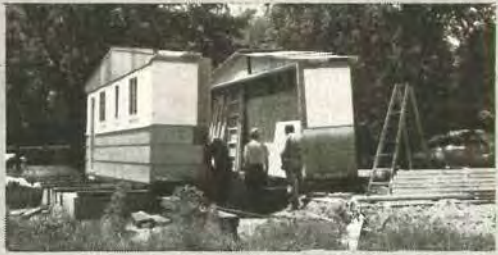
... Prefabricated panels and precut lumber stored in the units are used to complete the frame of the Knox-Bergstrom house when it arrives at site.
