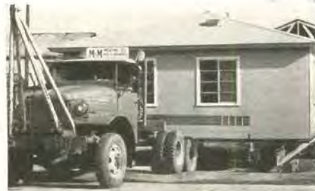
Right off assembly line, a Mobilhome is trucked to site, set on foundations . . .
