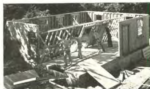
Walls are up at 11 a. m. Interior wall frames, often shipped in full-length sections, are easily tilted into place.
