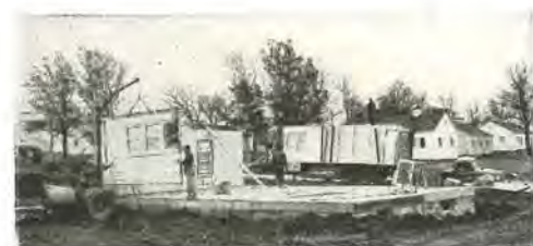
The truck tractor that delivers house panels has mobile crane that quickly swings panel off truck and into position.
